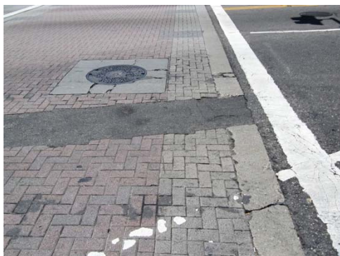
Decorative crosswalk treatments made of distinctive materials can become uneven over time.
