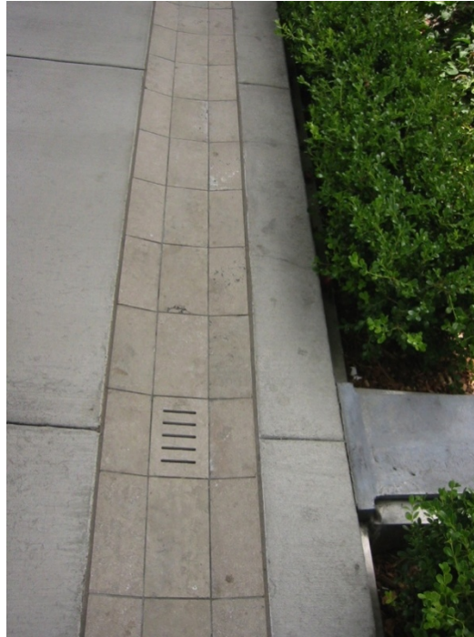
Constructed swale with drain (Credit: Stephanie Landregan)
